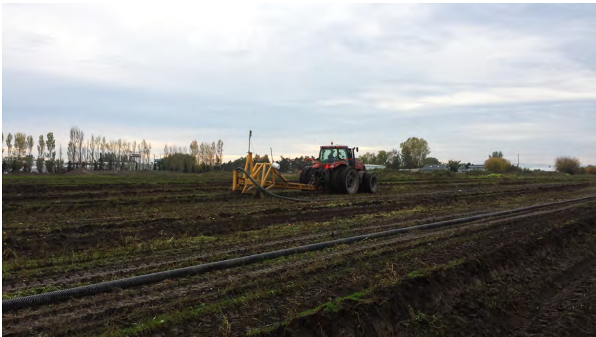
Figure 3 Tile drainage installation by collaborating farmer at the field-scale demonstration and research site
